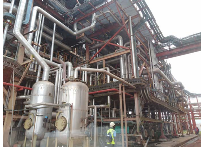
The Sunbird biomass factory to produce electricity
